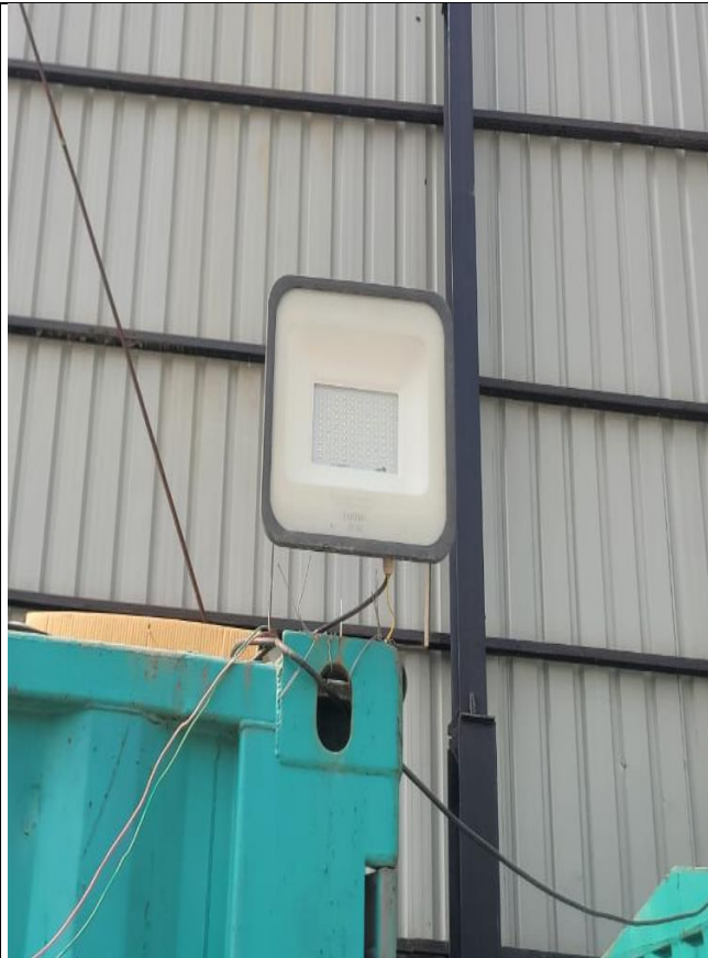
LED LIGHTS AT SITE
